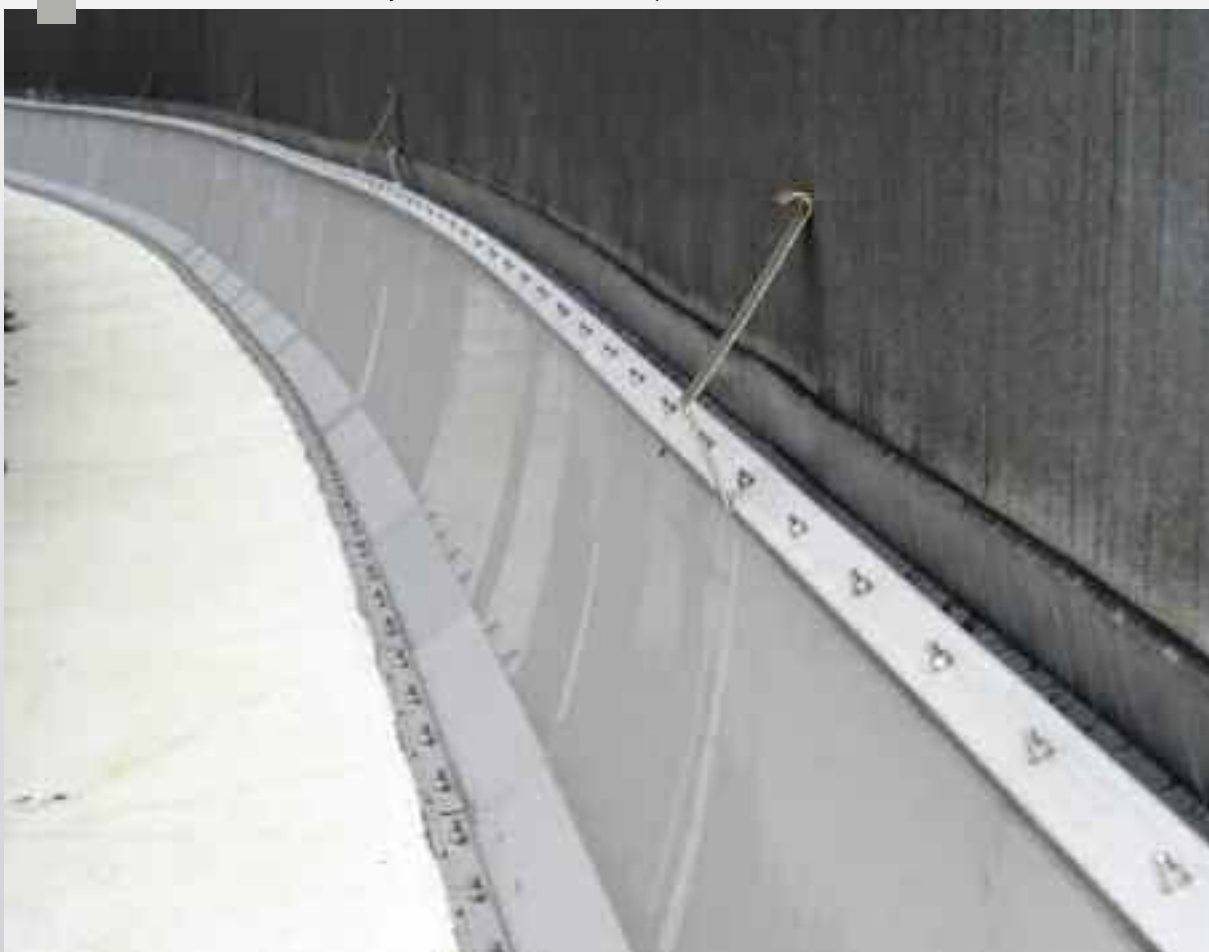
CTS30 BP CTS20L secondary seal after installation, top view
