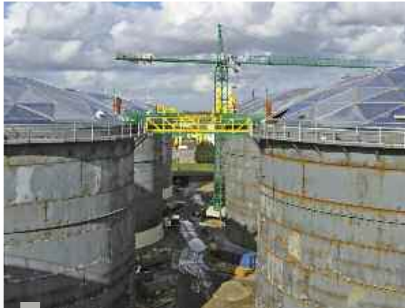
Dome project at Vopak Botlek as amongst the many completed projects in 2008 by CTS
