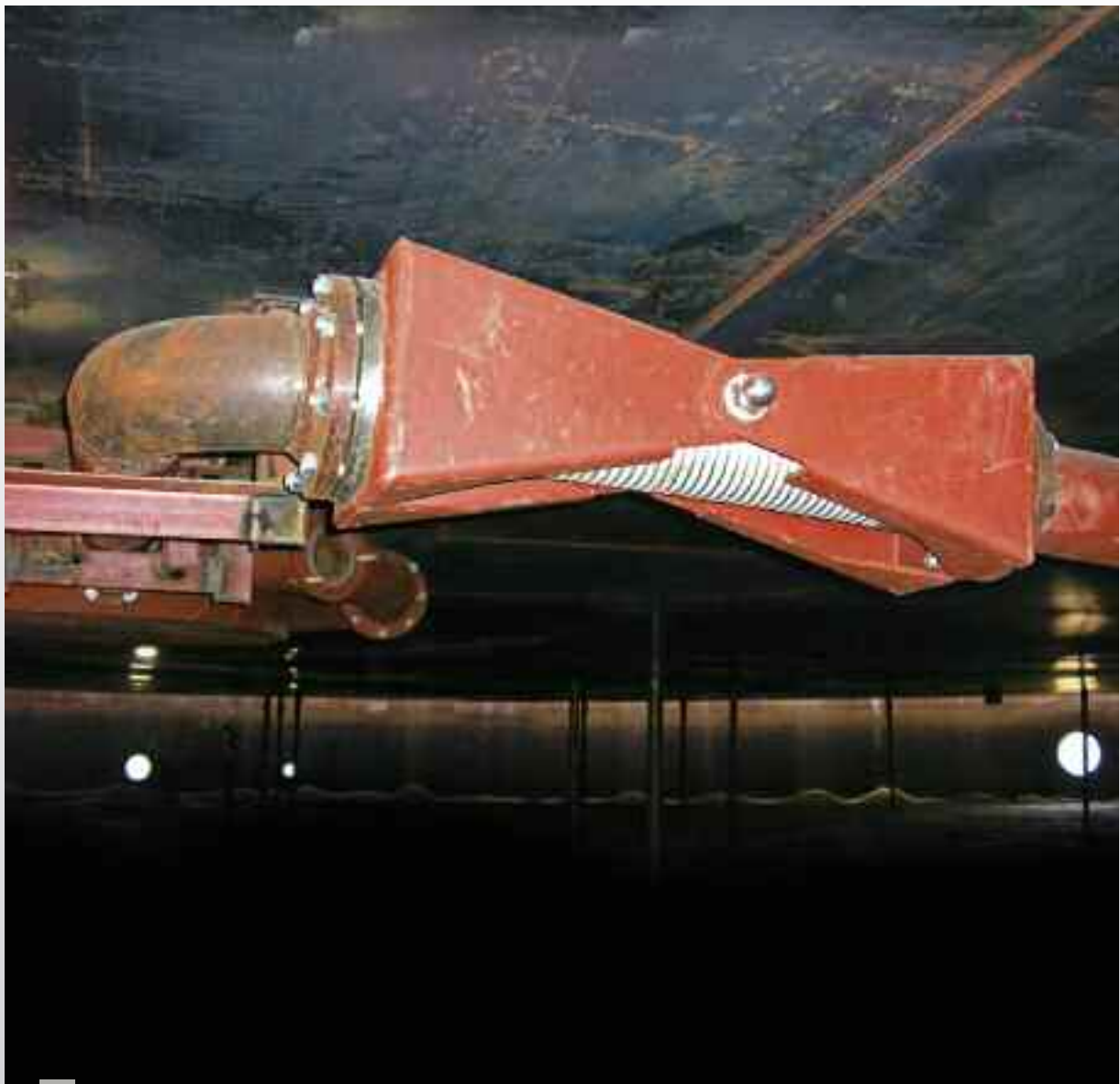
Drainmaster joint in tank drain line
