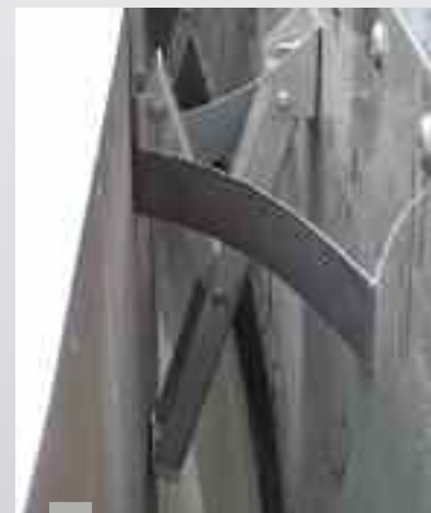
CTS1 scissor type shoe plate seal hanger assembly and shoe plate prior to vapour barrier installation
