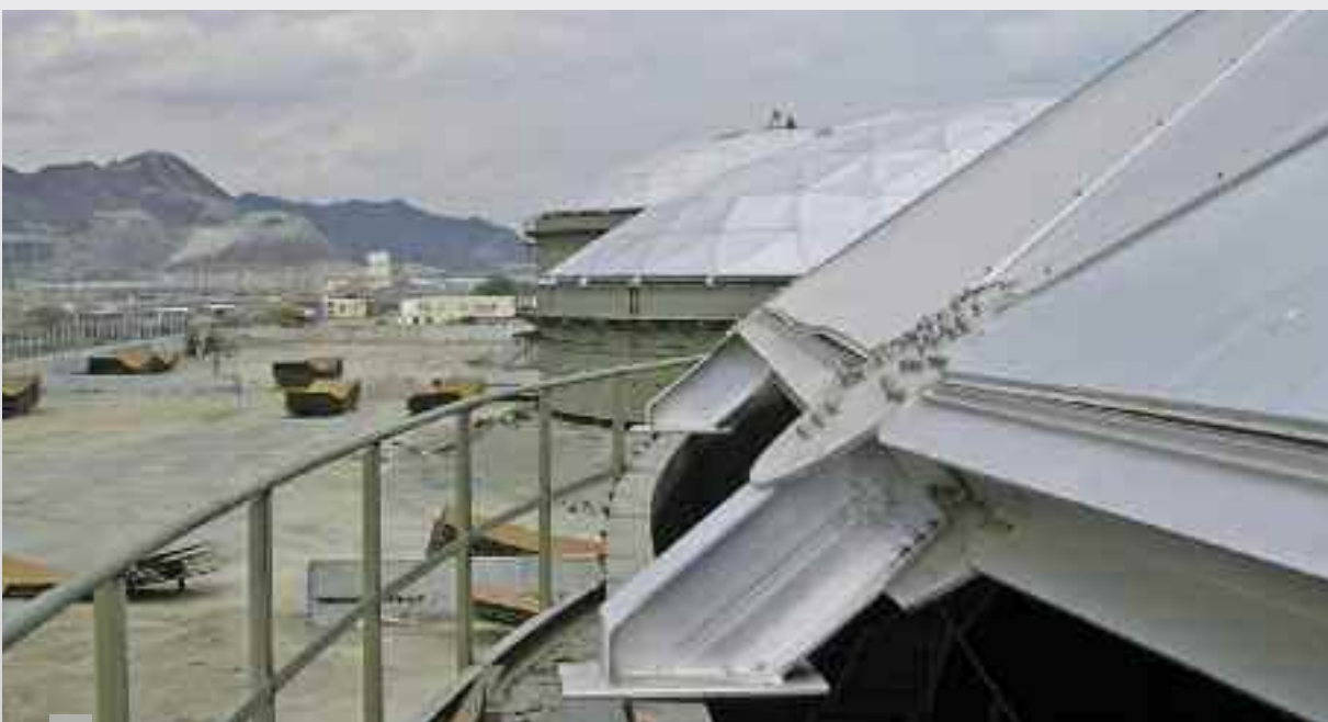
Vitol UAE Domes were lifted on early, and jacked along with the remainder of the tank shell rings added
